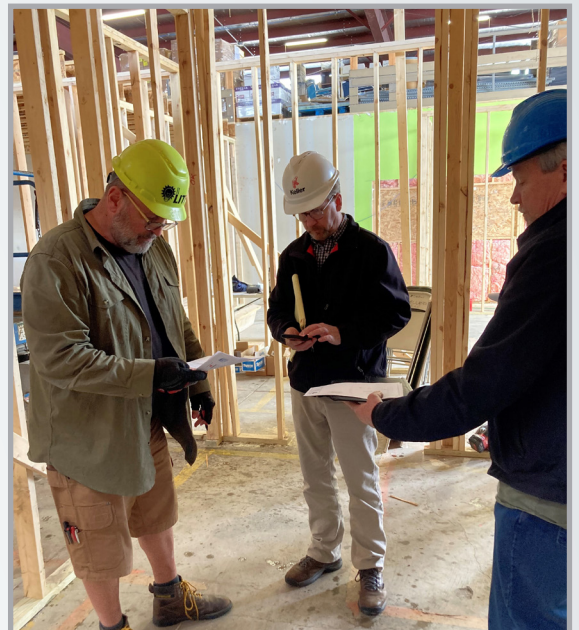
Subcontractors review the electrical plan for the renovated interior at Good News Project
